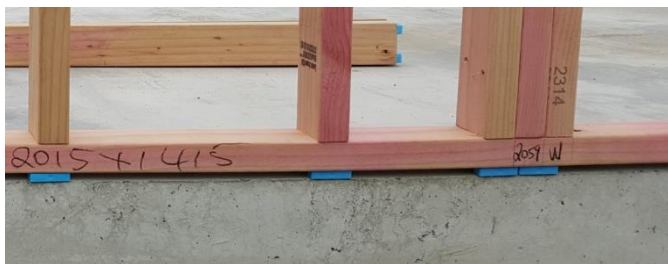
Lintels over 1400mm require 2 packers each side, Lintels over 4000mm require 3 packers each side.
